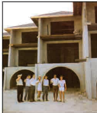
The men behind Villas Pappagallo (l to r) Gordon Alexander, David Challiee, Ken Spraggon, John Elliott, Heber Arch, Peter Fedele and Adrian Bertolotti celebrating roof on Phase II. Completion scheduled for February, 1982.
